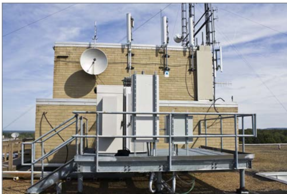
Figure 1: Typical Wireless Base Station with BBU
