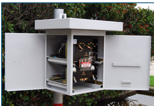
Figure 6. | Image of a typical cathodic protection rectifier
