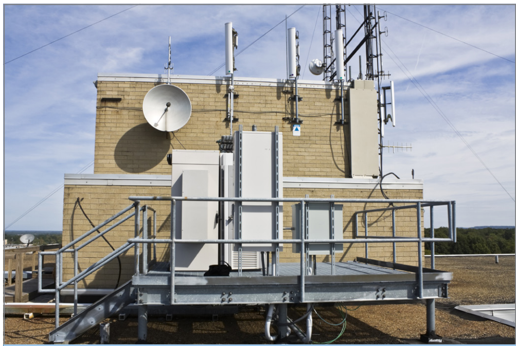
Figure 1: Typical Wireless Base Station with BBU
